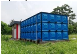
Gambar 4. Bak penampung ( reservoir )
